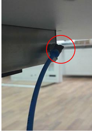
Figure 34.9 Gas line connection under the tabletop
