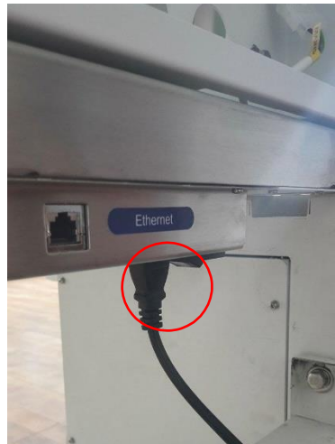
Figure 34.8 Main power connection in the Multi-zone ART Workstation
